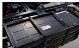
BATTERY 3 72 kWh (3 x 24 kWh each)
